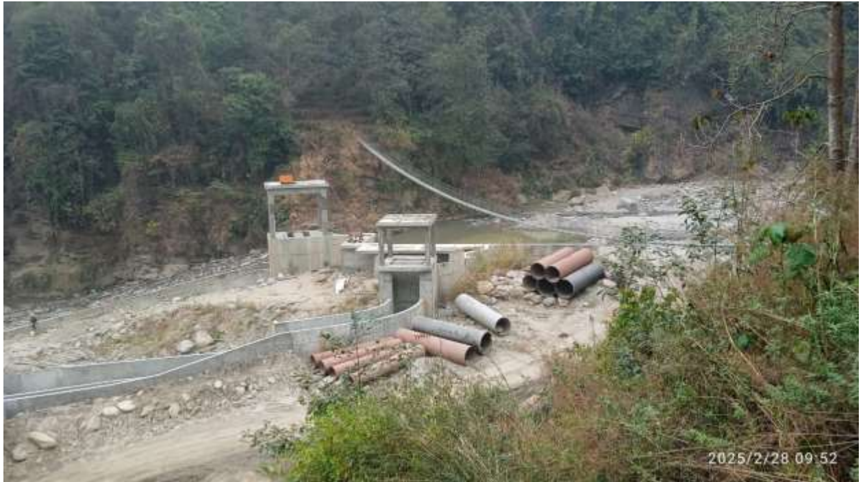
Figure 1: Overall Headworks area.
